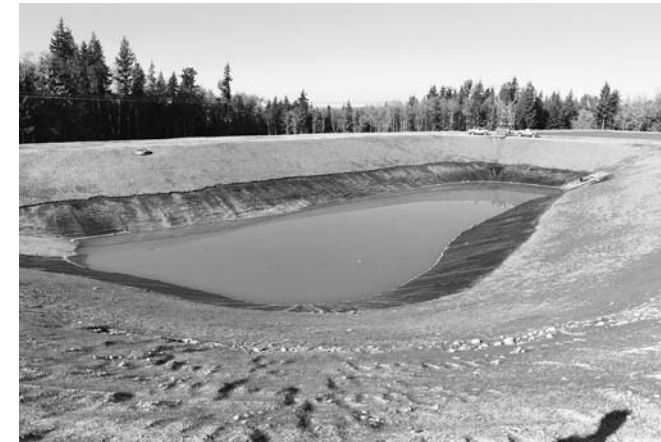
Lined sediment basins are used to collect runoff from disturbed areas on construction sites and allow heavier solids to settle out.
