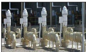
Figure 14 - Recovery well pumps
