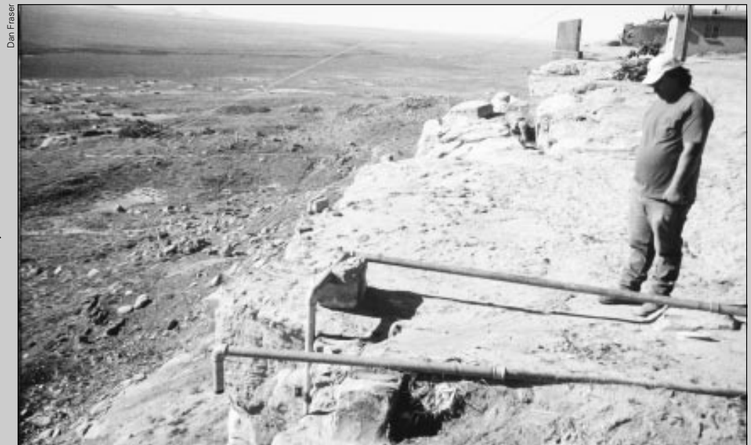
Chuck Villa, water system operator, looking down at the exposed transmission main ascending the face of the cliff.
