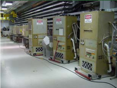
Ring RF equipment in the tunnel
