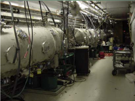
Cryomodules installed in the Linac Tunnel
