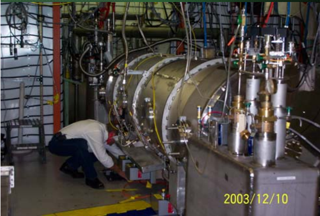
Cryomodule M-4 in the Test Facility
