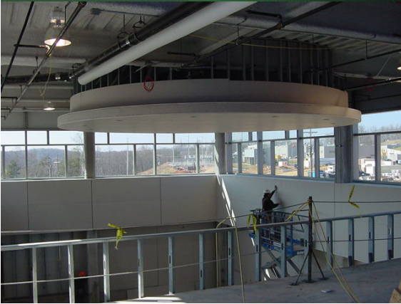
CLO control room
