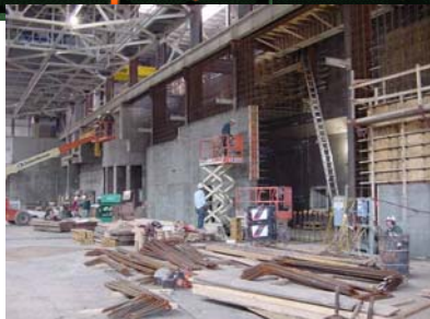
Target Hot Cell wall
