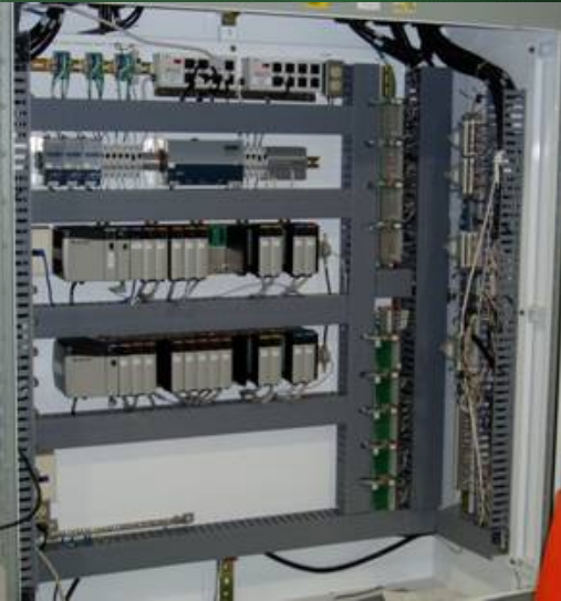
4.5K Cold Box Integrated Control System
