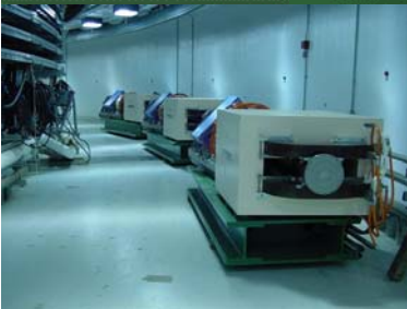
Ring Half-Cells in the Ring Tunnel
