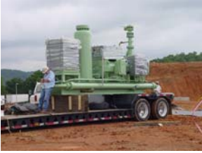
Compressor skid for the Target building arrives on site
