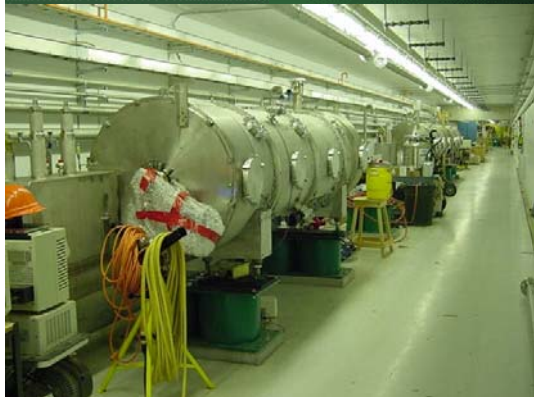
Installed cryomodules 1,2 and 3
