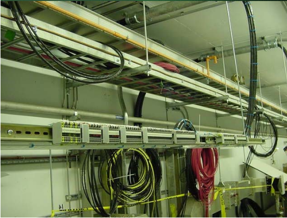
Controls cable trays
