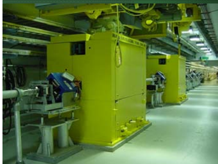
HEBT Collimators installed
