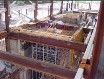
Target Hot Cell ceiling
