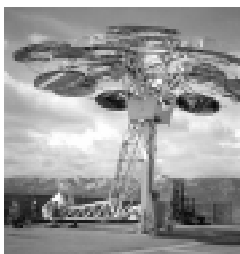
Workers install the Stirling engine on dish/Stirling system at NREL. See page 2.
